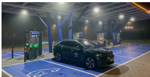
The overall impression counts: Our evaluation includes the signage and marking of the charging parking spaces, but also comfort and safety aspects such as lighting and camera surveillance.
