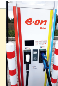
Outage: At two locations, charging was not possible.
