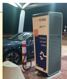
Reliable energy: The EnBW columns worked stably.
